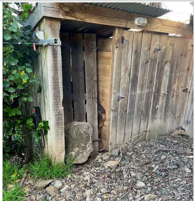
North Piha - Rockfall (debris)
